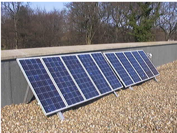
Figure 6: Photovoltaic array for testing the MPP algorithm (10 series connected 70 Wp modules).
